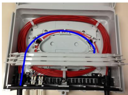
main cable => trays câble principal => cassettes
