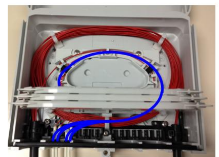
trays => drop cables cassettes => câbles branchement
