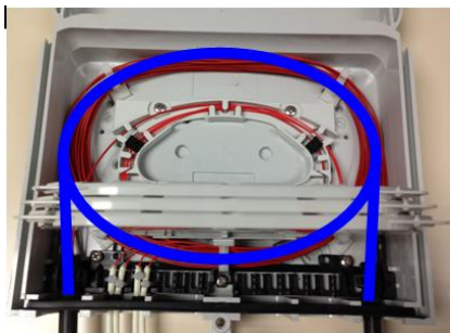
main cable routing circuit du câble principal
